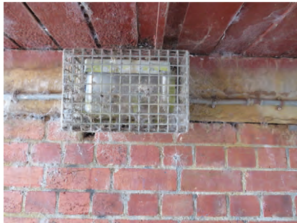
Is this the light installed in the Middle Park underpass following the Council meeting?
